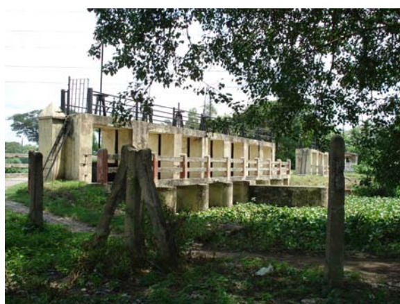
Lock gate in fishery feeding canal
